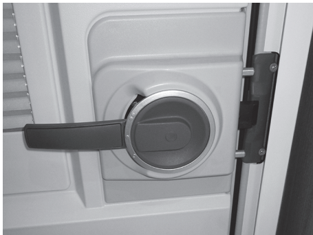
Fig. 15: Closed but unsecured door lock
