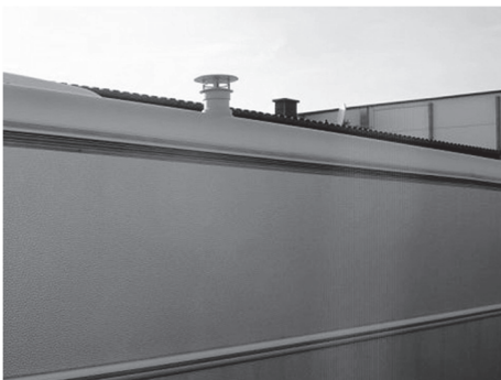
Fig. 82: Exhaust gas stack of the gas heater
